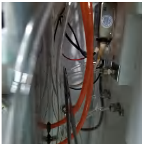
Figure 4-7 the Oxygen Flow Meter to the Oxygen Valve the gas pipe
